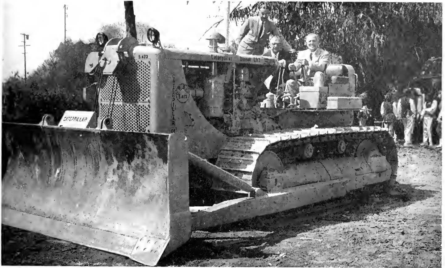
Robert E. McClure, member of the California Highway Commission, left, and Mayor R. C. Miller of El Monte watch as Governor Knight manipulates the controls of a bulldozer used to break ground for a new section of the Ramona Freeway in Los Angeles County
